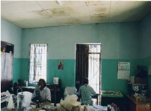
Leaky Roof -- Before
